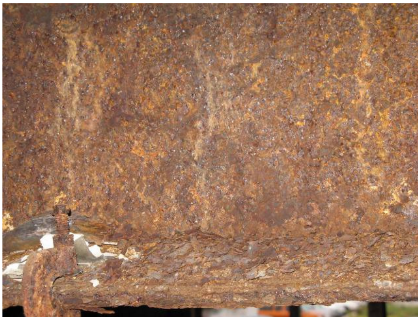
Photo #29: Heavily corroded bottom flange of steel girder below mezzanine slab
