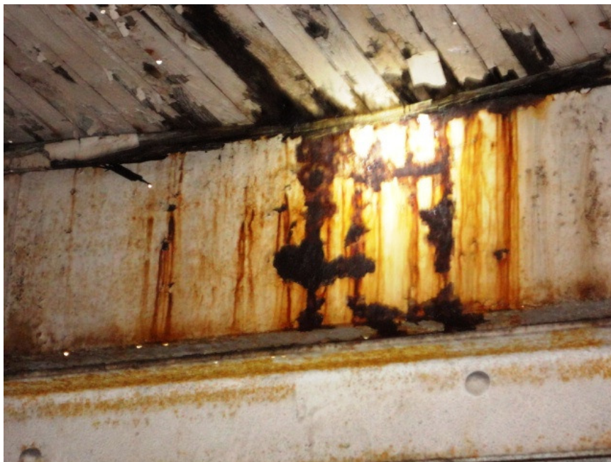
Photo #21: Typical roof leak causing corrosion on top flange of girder in Addition
