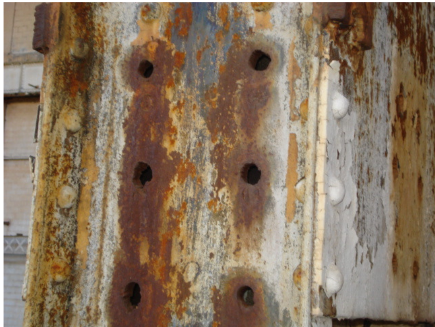
Photo #25: Typical missing rivets on column along gridline Ds
