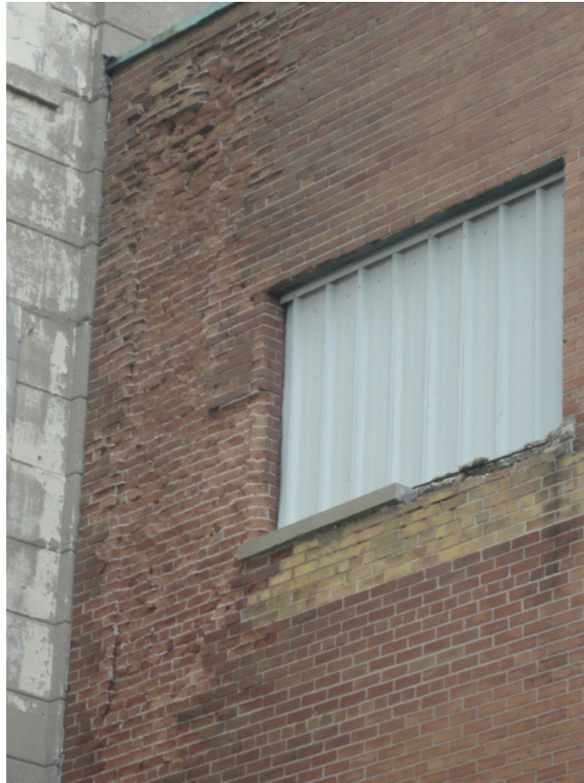
Photo #48: Deterioration of masonry wall at junction with existing wall
