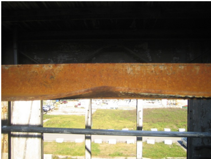
Photo #19: Typical dent/kink in truss member
