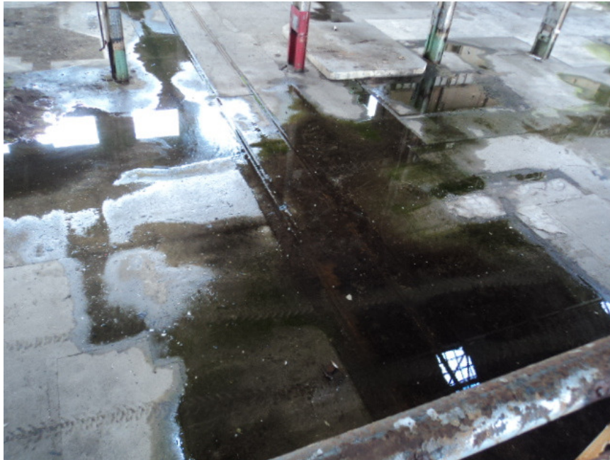
Photo #44: Slab-on-grade area of differential settlement
